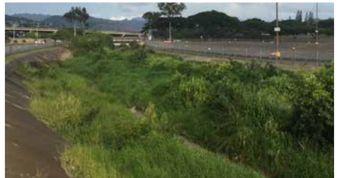
Halawa Stream is channelized as it bisects the Aloha Stadium parking lot
